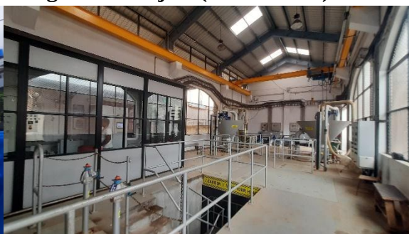
Bambalapitiya Pumping Stations
