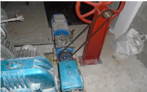
Gate hoisting system of Alikota Ara project
