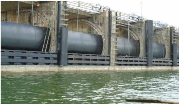
Water control gates at Rajangana reservoir
