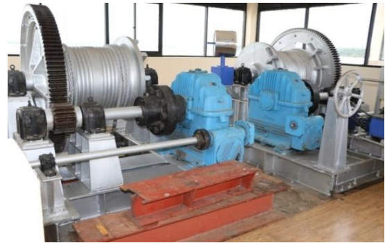
Gate hoisting system at Deduru Oya reservoir
