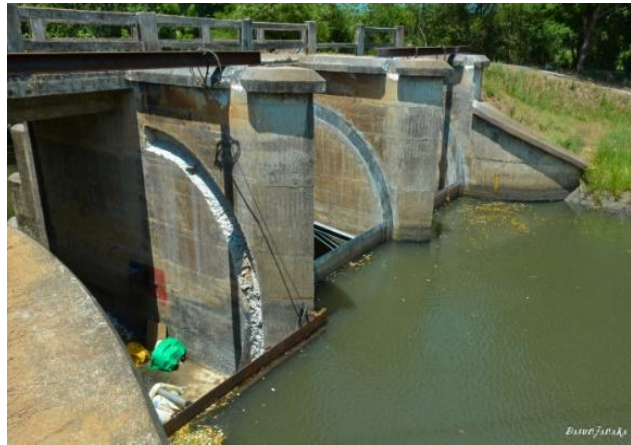
Galamuna project water control gate
