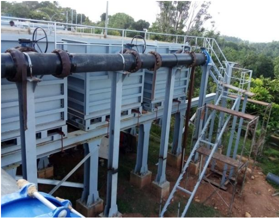
Hapugala Water treatment plant
