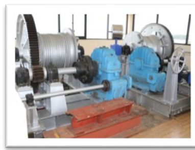
Gate hoisting system at Deduru Oya reservoir
