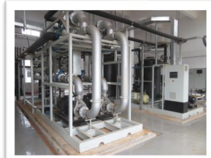
Leachate Treatment Plant
