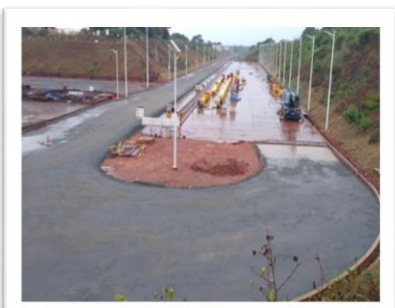
Gantry Crane Platform
