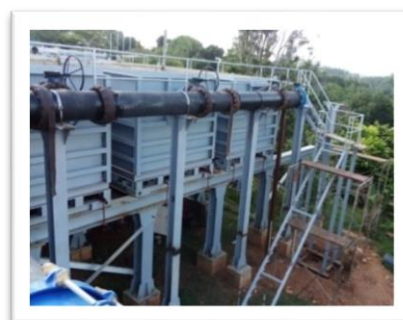
Hapugala Water treatment plant
