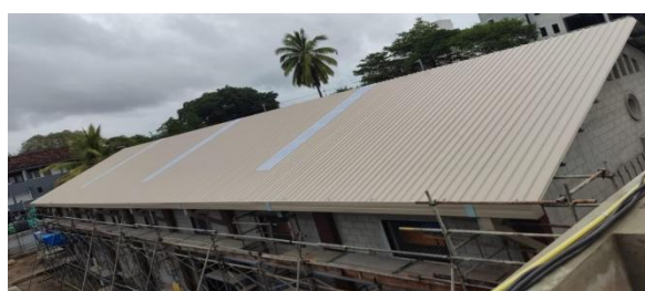
Borella Pumping Station
