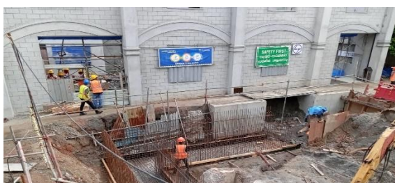
Thimbirigasyaya Pumping Station
