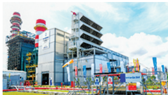
(Commissioning of LNG Plant – Kerawalapitiya)
