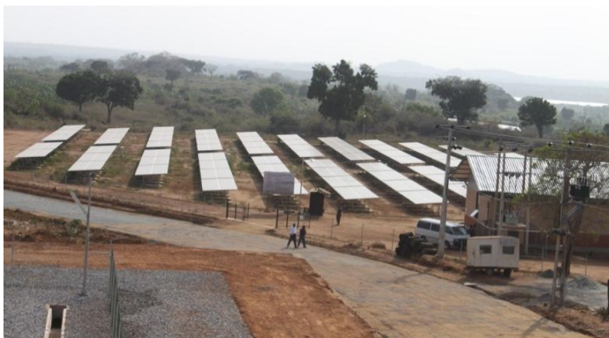
Figure 3.5: 500 kW solar plant
